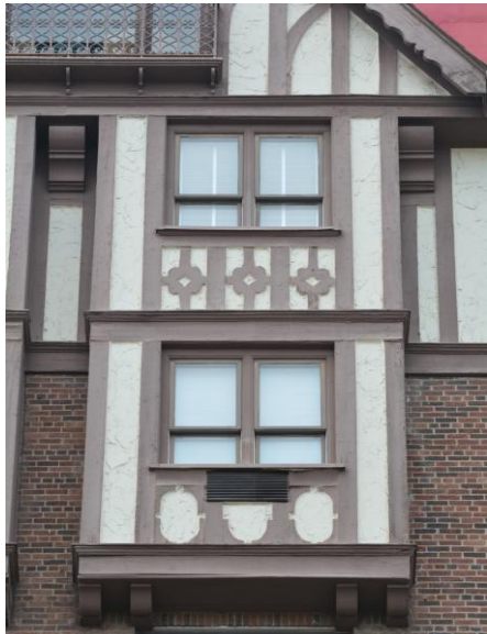
NON-ORIGINAL DOUBLE HUNG WINDOWS (TYPE 2)
